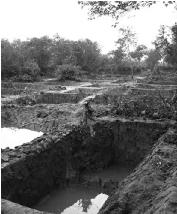
Fig 6.4. Holes dug for embankment maintenance, Colony Para, Sagar Island. Photo by author.
