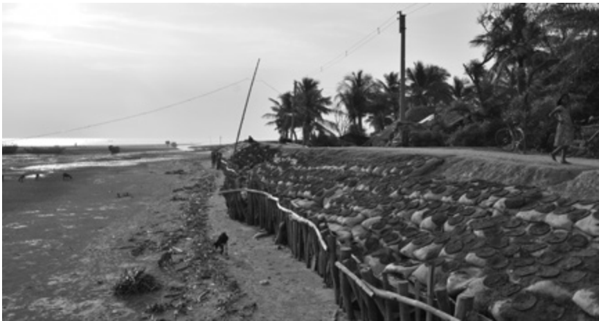
Fig 6.3. Embankment made of sandbags, wood, and mud, Sagar Island. Photo by author.
